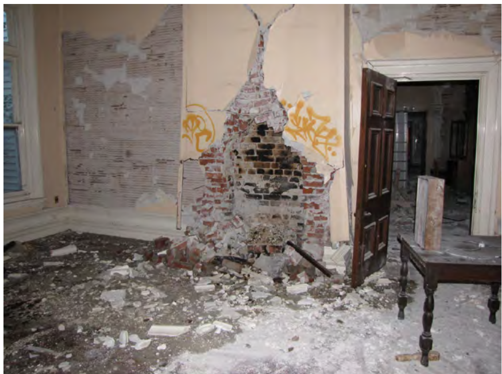
► Fig. 25. Brick fireplaces have collapsed (Source: W. Clark, 24/11/2015)
