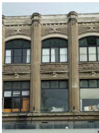
◀ From left to right: Fig. 5. McKenzie and Willis building post September 2010 earthquake (Source: Carole-Lynne Kerrigan, n.d.) Fig. 6. McKenzie and Willis building post September 2010 earthquake (Source: Carole-Lynne Kerrigan, n.d.)
