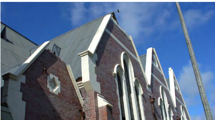
Fig. 6. September 2010 earthquake damage to northern gables (Source: CCC, 27/1/2011)
