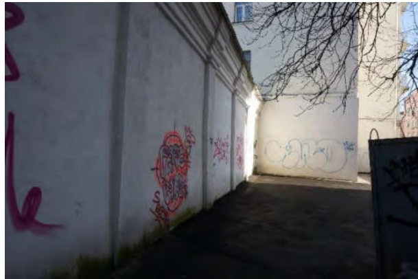
Detail of the surrounding wall with graffiti damage
